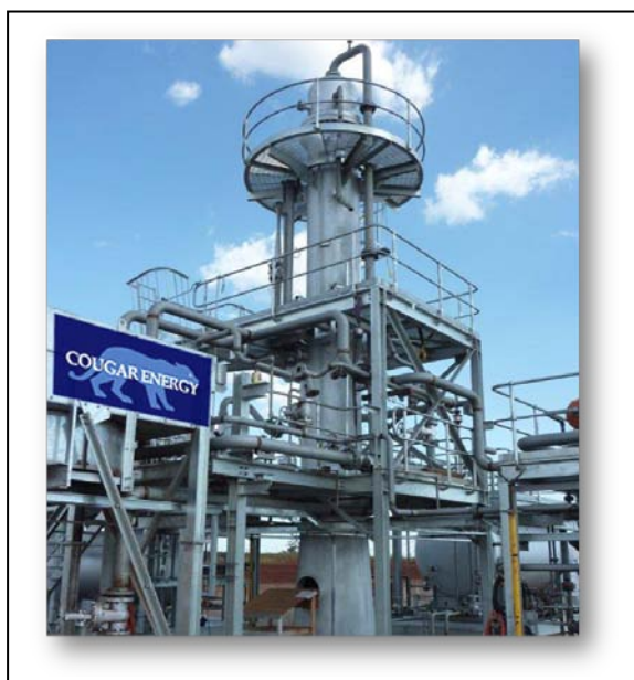
Kingaroy Gas Processing Plant
