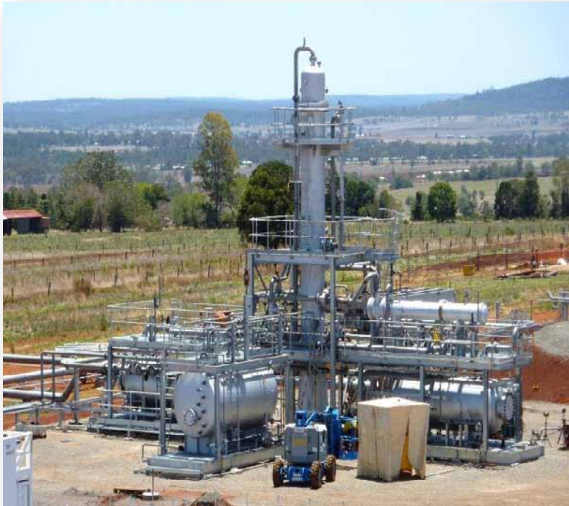
GAS PROCESSING PLANT
